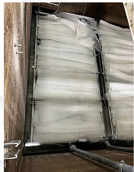
WavTex Modules Upon Installation in Aerated Tank (note the media sheets are buoyant and rise with the water level)
