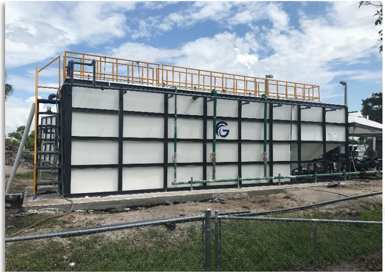
Above: Galene FRP Vessels with WavTex modules. Modules were installed in the aerated portion of the vessels.
