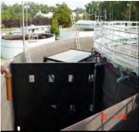
Aerobic Selector Zone and IFFAS Frame
