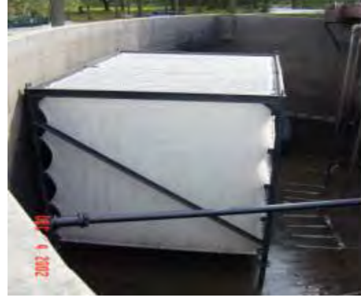
IFFAS Frame Showing Aeration Headers
