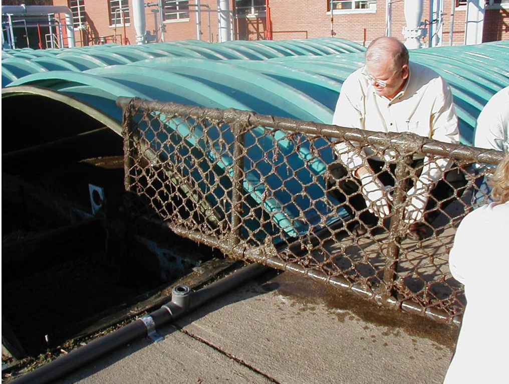
Figure 8: Sample rack of BioWeb media removed for observation in 2004 (Photo courtesy of Freese and Nichols)
