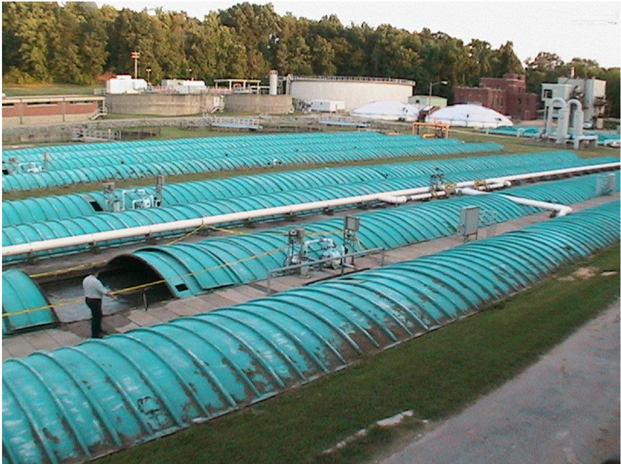
Figure 1: North Buffalo Creek WRF overview, including aeration basins with covers
